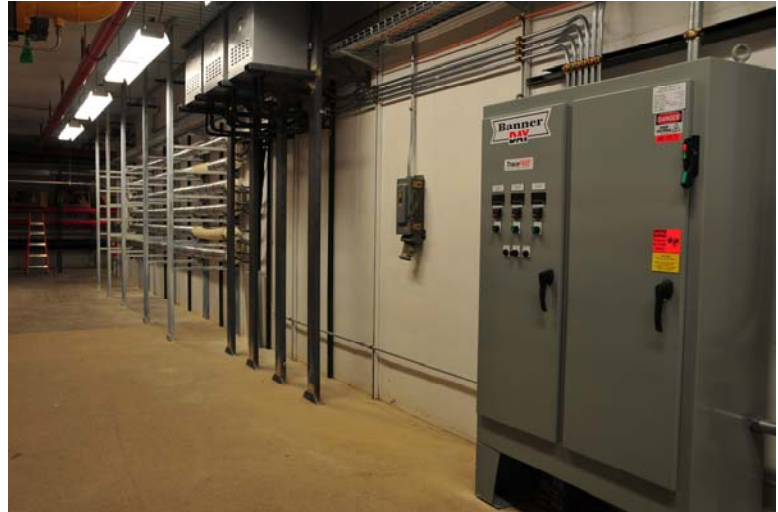
Total System View (2)
