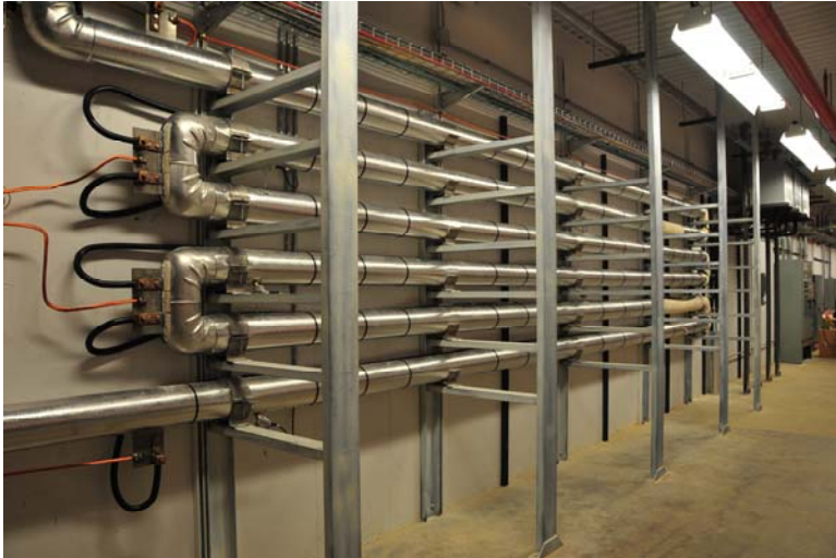
Total System View (1)
