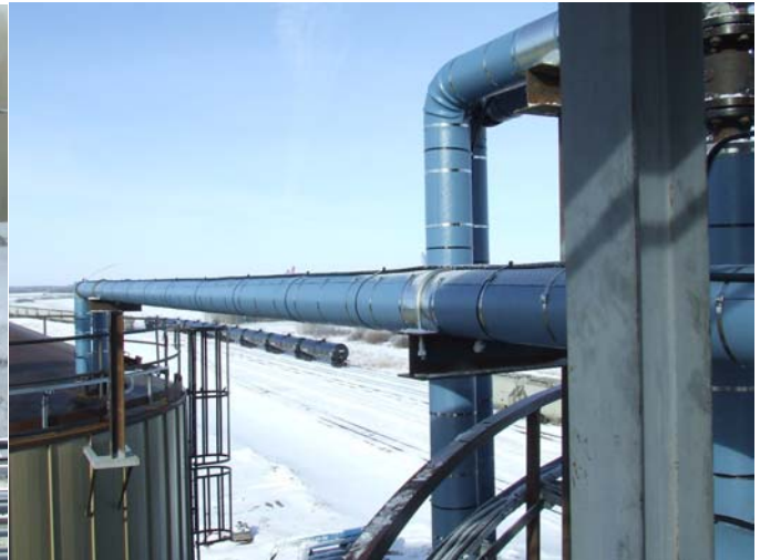
Two (2) TraceFREE™ heated lines serving a Load-Out Tank.
