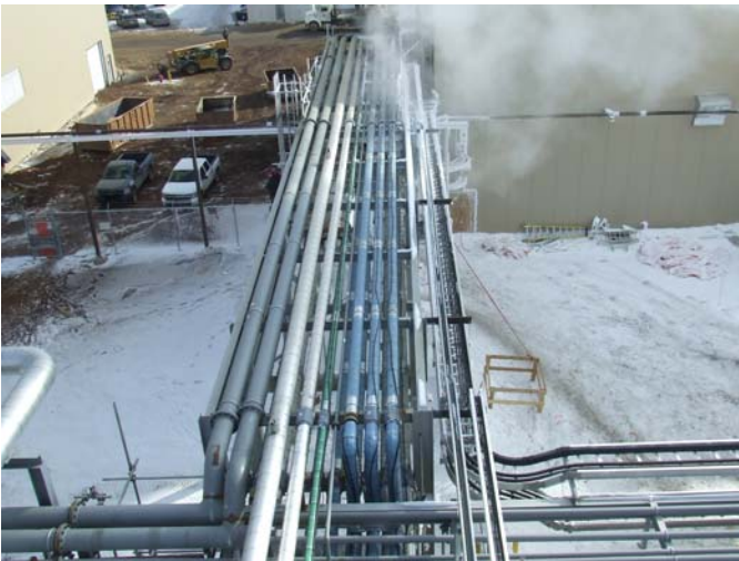
TraceFREE™ heated lines installed on Pipe Bridge.
