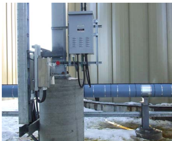
Impedance Transformer with Disconnect
